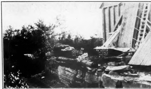
View of crushing plant showing location of crusher and boxes made of boiler sections in which stone is moved by derrick
